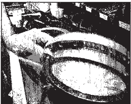
4 Working on the operating handle portion of the valve to which the old sleeve is still attached.
