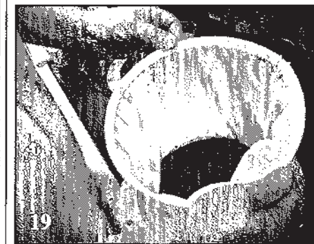
19 Ease the ends of the wires around until they align themselves with the seam on a fabric sleeve or small reinforcing patch on a rubber sleeve.
